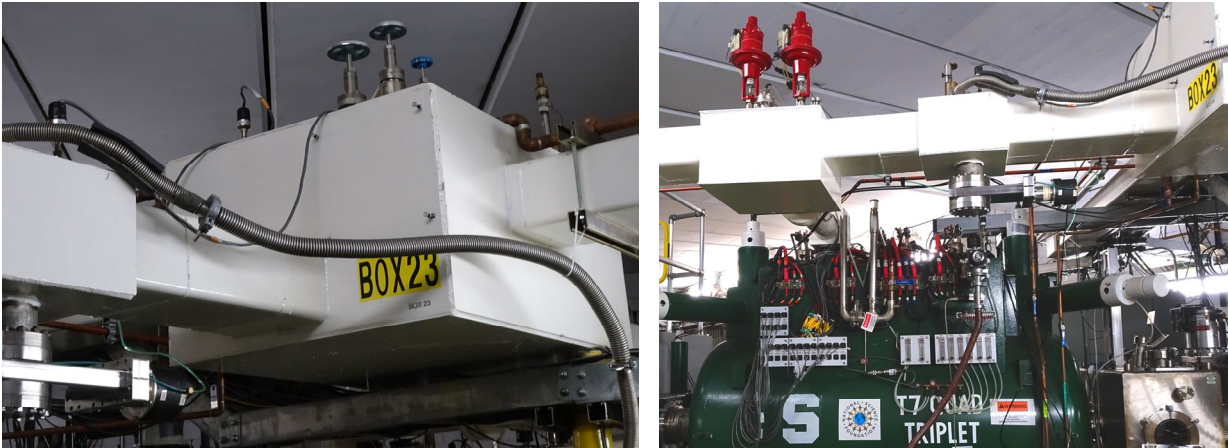
Figure 11-2 (a) NSCL Box 23 similar to proposed HRS Branch Box 2; (b) NSCL local valve box and transfer line section similar to proposed local HRS cryogenic boxes and transfer line
